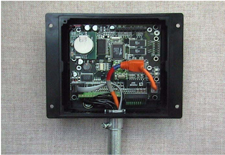
Figure B-10. Rear View of Intellicom with Outer Casing Showing Wiring from Conduit
