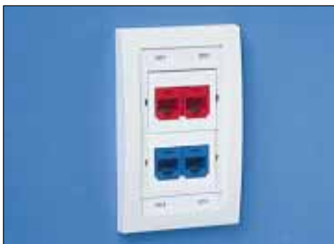
Network Systems Labeling
