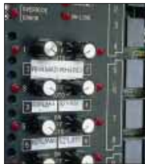
Label switches, relays and other devices
