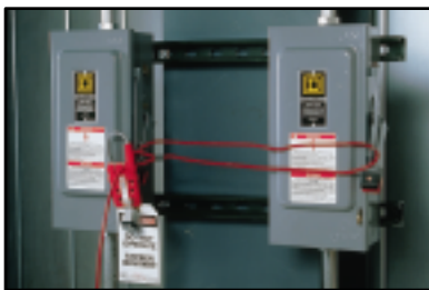
Lockout Single or Multiple Disconnects
