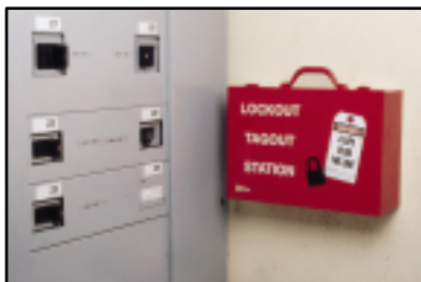
Mount close to power and distribution panels
