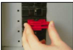
Turn switch to off position. Place lockout over desired switch.
