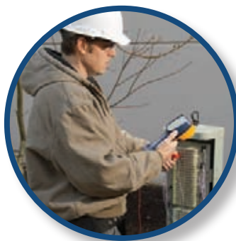
Cross Box or Serving Terminal
