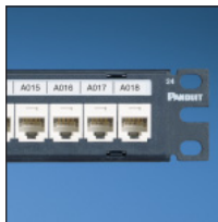
Patch Panel Labeling
