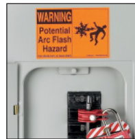
Safety Sign Labeling
