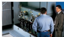
COOPER Power Systems
