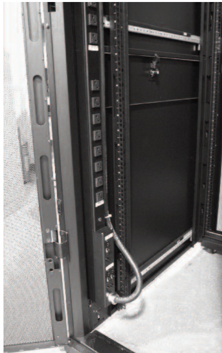
Power Commander Plus High Current Power Distribution Unit shown mounted in an IT cabinet.
