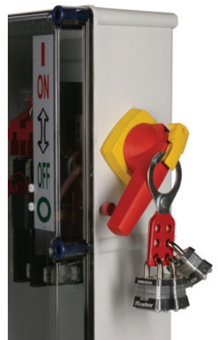
Halyester switch can be padlocked in the OFF position by extending handle hasp.
