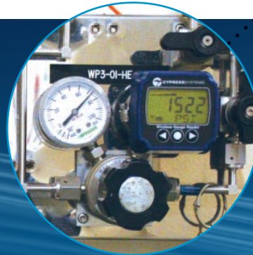
INDUSTRIAL MONITORING AND CONTROL
