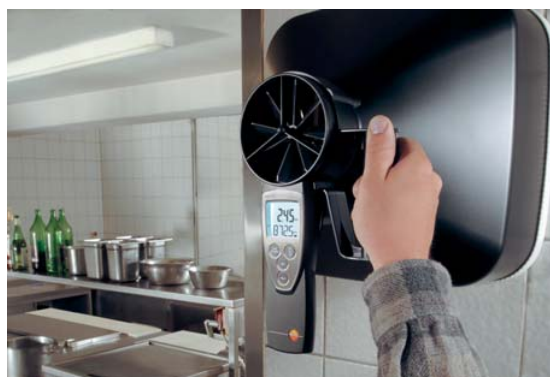
Using the testo 417 to monitor the exhaust air at a wall-mounted ventilator
