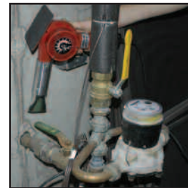
Thaw Frozen Pipes
