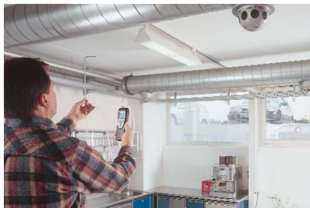
Measuring outlet air
