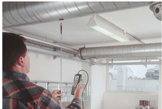
Using the testo 416 to set air input in a kitchen
