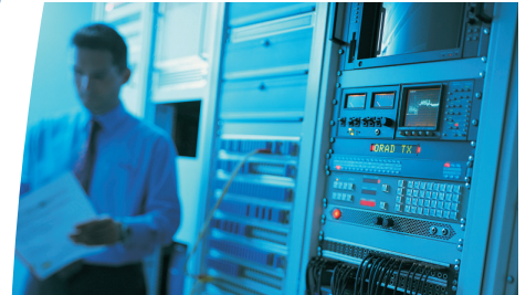
Servers, data storage and network equipment.
