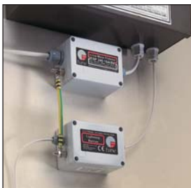
Security alarm panel with ESP TN/BX (bottom) providing protection from transient overvoltages on the dial-up telephone line. Note how the ESP TN/BX is earthed via a bond to the ESP 240-16A/BX (top) installed on the mains power supply to the panel
