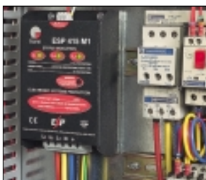
ESP 415 M1 installed within a control panel on the mains input to protect the panel's control systems. Note the remote indication connection (top of protector).
