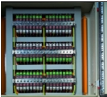
Three rows of protectors, inside a control cabinet, each installed on a CME 16 combined mounting and earthing kit.
