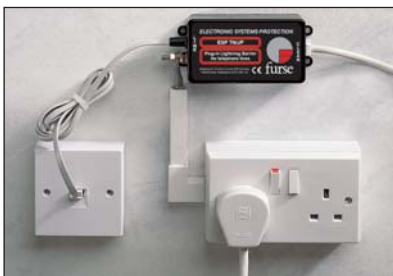
The installation above clearly shows a protector installed with a short earth connection to the same earth as the equipment it's protecting
