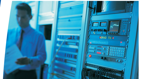
Servers, data storage and network equipment.
