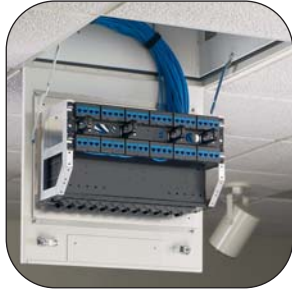
Zone Cable Boxes
