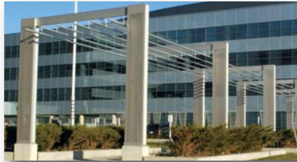
188 Perforated stainless steel plates are bonded to I-beams with 3M™ VHB™ Tapes as they replace rivets or screws for a smooth surface envisioned by the architect.
