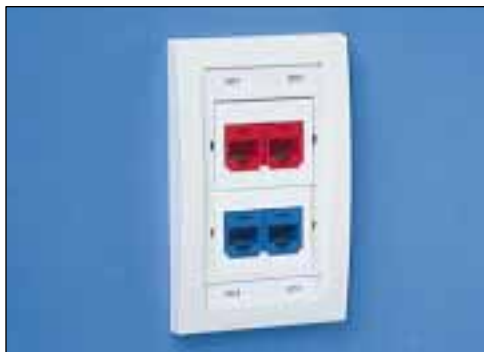
Network Systems Labeling
