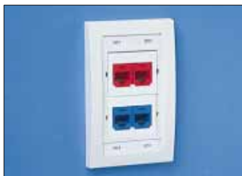
Network Systems Labeling
