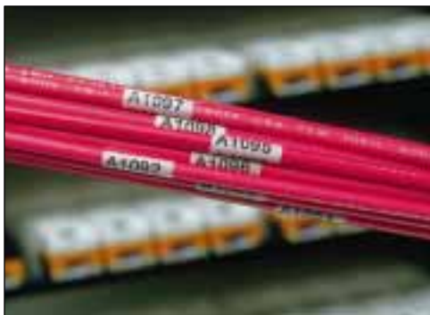
Wire and Cable Identification
