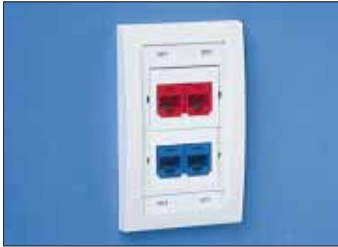
Network Systems Labeling
