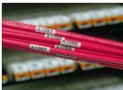
Wire and Cable Identification
