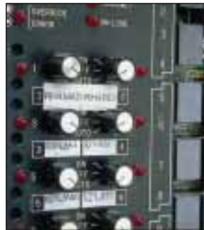
Label switches, relays and other devices
